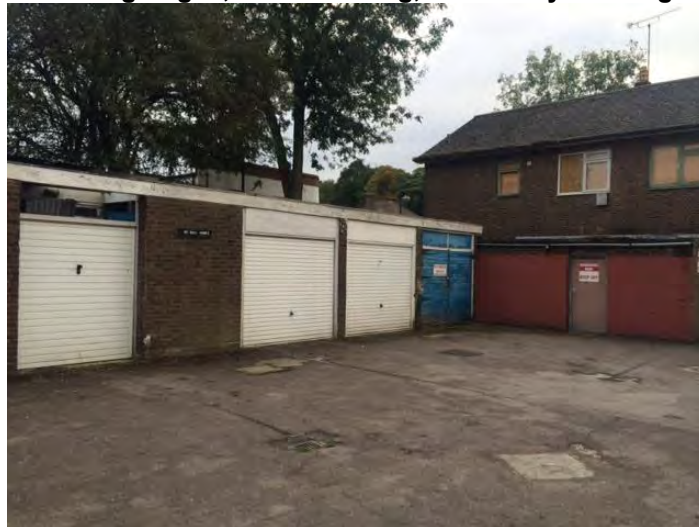
Figure 3: Northern gable end of the two storey building showing small gaps under the soffits
